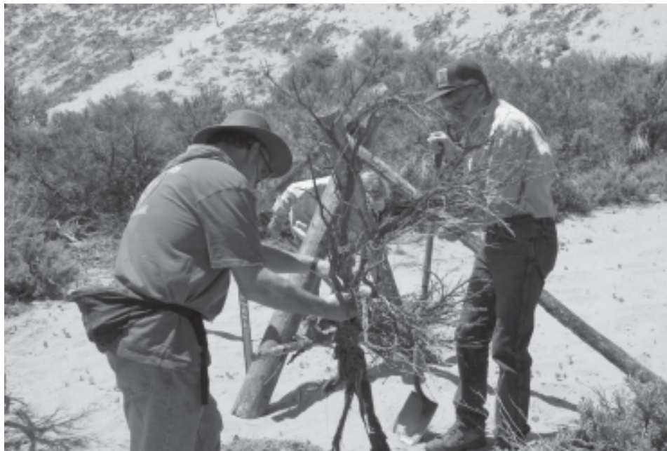
LUV volunteers assist the BLM in building a barrier to illegal OHV incursions at Moquith Mtn Wilderness Study Area.
