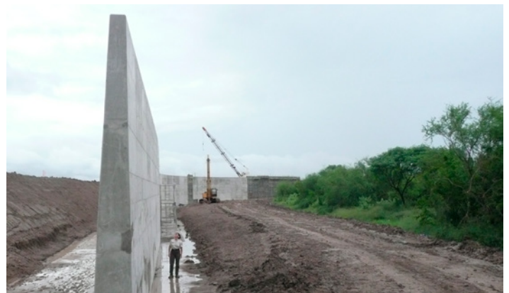
LEVEE BORDER WALL DURING CONSTRUCTION THROUGH THE LOWER RIO GRANDE VALLEY NATIONAL WILDLIFE REFUGE. PHOTO: MATT CLARK, DEFENDERS OF WILDLIFE
